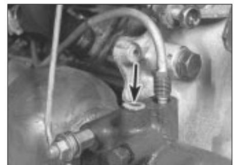
4.4 Disconnecting the rigid pipes from the pressure regulator. Note the plug inserted into the vacated port (arrowed)
